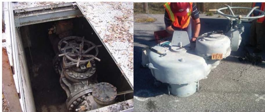
FIGURE 4-11 PACIFIC GAS AND ELECTRIC COMPANY EXISTING MANUAL VALVES REQUIRING REPLACEMENT
