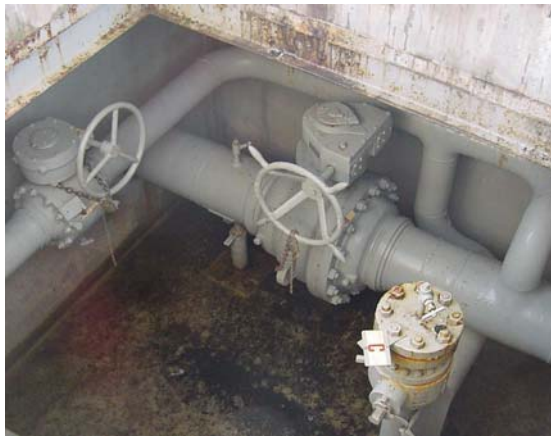
FIGURE 4-9 PACIFIC GAS AND ELECTRIC COMPANY MANUAL VALVES INSTALLED IN A VAULT
