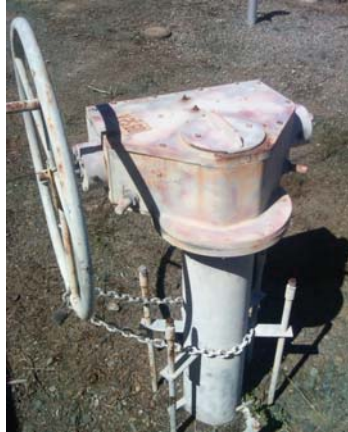
FIGURE 4-10 PACIFIC GAS AND ELECTRIC COMPANY BURIED VALVE WITH MANUAL GEARING INSTALLED ABOVE GROUND
